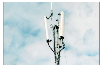
Telecoms: asset management
